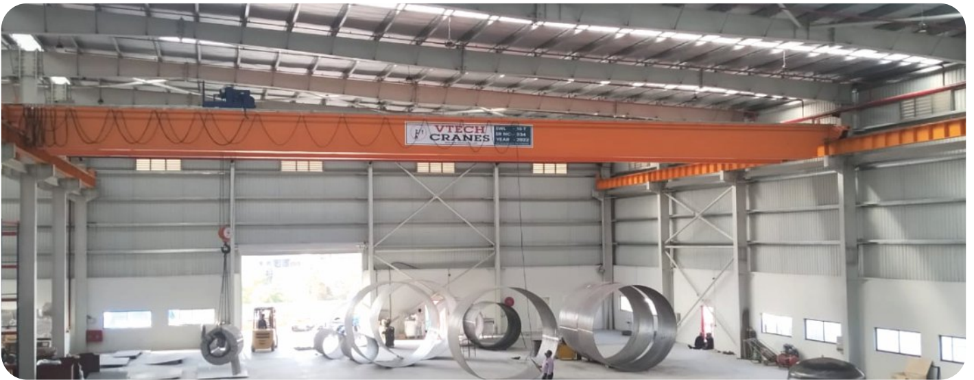
DOUBLE GIRDER EOT CRANE (DGEOT)
